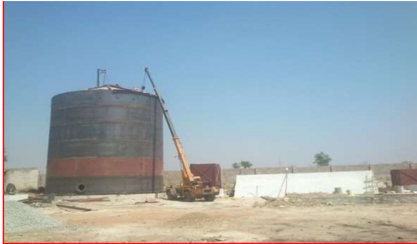
Anaerobic Reactor Shell-2
