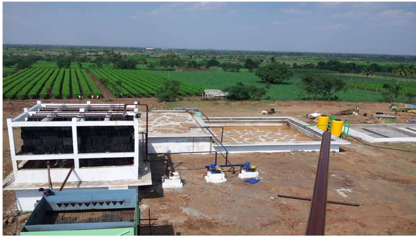
SSWL- Two stage Diffused Aeration : A new process launched at that time
