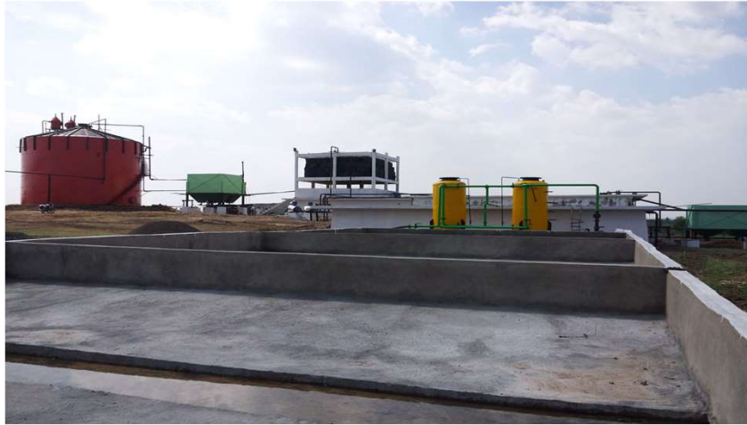
2. Shiraguppi Sugars Ltd , Miraj , Maharashtra: Digester & ETP: Turnkey project
