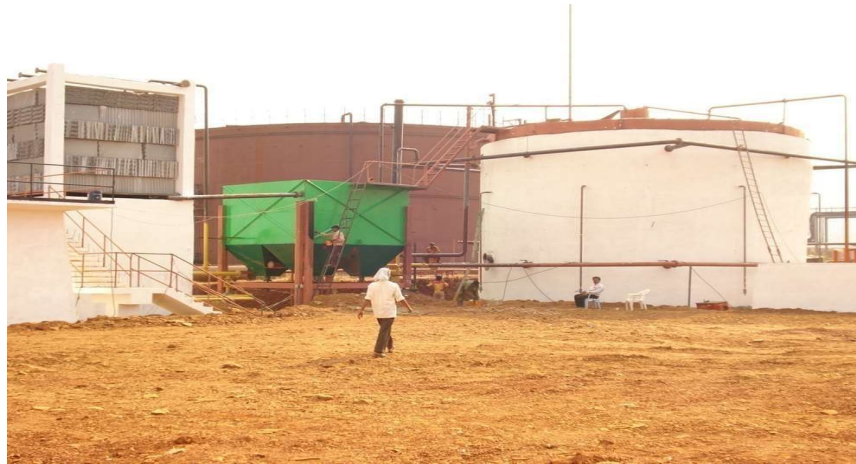
1.Vijay Nagar Sugars Ltd ; Gadag –Karnataka- Digester & ETP-Turnkey Project
